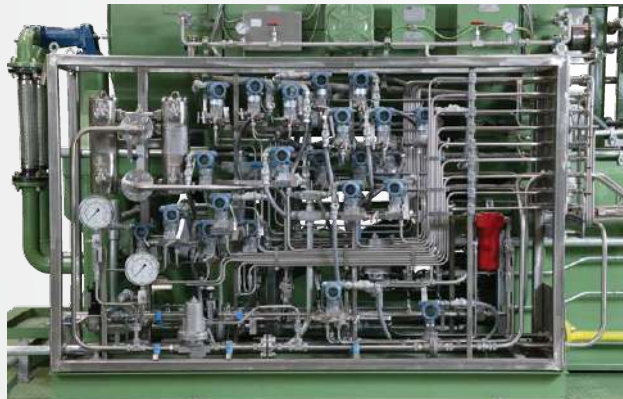
Gas seal transmitter rack with 2-of-3 voting, seal gas filtering and purge gas filtering
